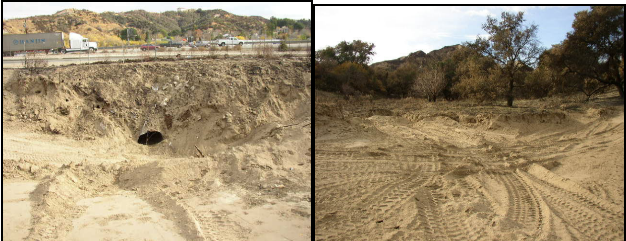
Dozer work next to/and upstream of a The Old Road culvert (19Dec2003).
