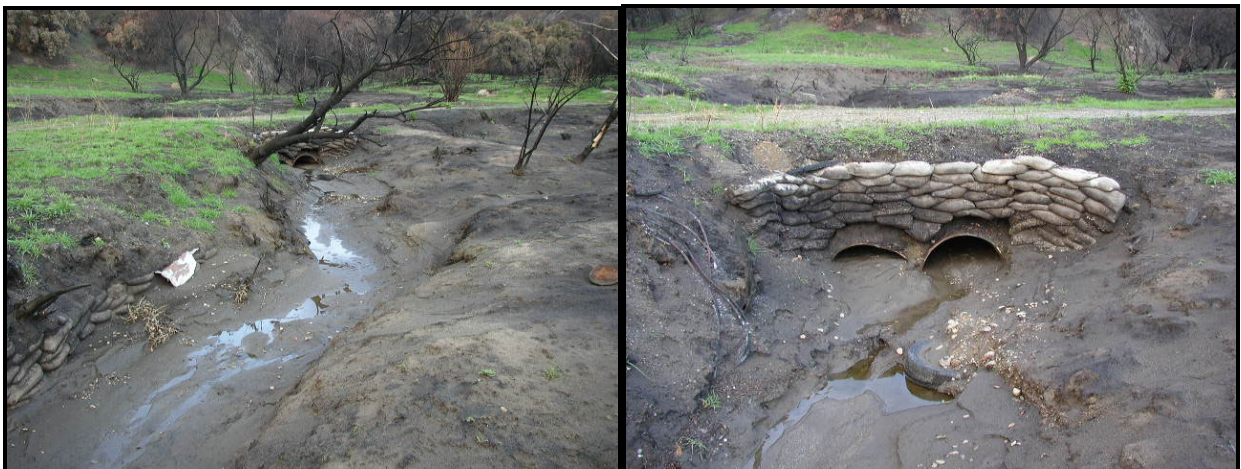
Sandbag bank stabilization and an old culvert crossing on Lyon Canyon Creek (23Feb2004).
